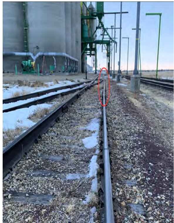
Figure 3. Track alignment issues
