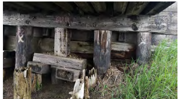
Figure 2. East abutment existing piles 2, 3, 4, 5 prior to bridge repair and polyurethane foam injection. Note the soil erosion near the bottom of the photo.
