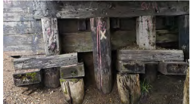
Figure 1. East abutment existing piles 1, 2, 3 prior to bridge repair and polyurethane foam injection. Note the granular falling through the undermined backing planks.
