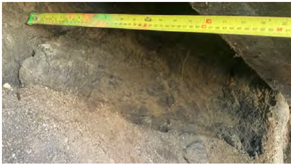
Figure 5. Backwall soil void on East abutment wall measured approximately 12 inches following backwall and pile repairs and prior to polyurethane foam injection.
