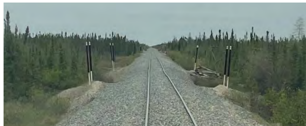
Figure 6. Typical thermosyphon installations in the Charlebois area.
