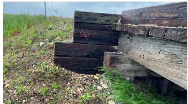
Figure 3. Damaged backing planks on the West abutment wall prior to bridge repair.
