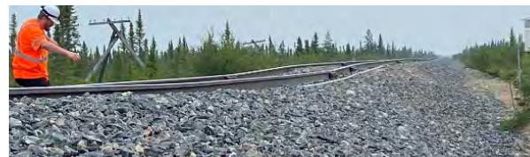
Figure 1. Typical Sinkhole on the HBR.
