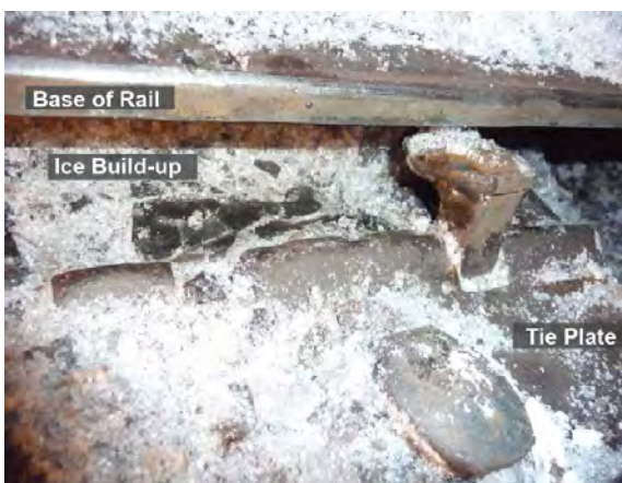
Figure 1. Ice buildup on tie plate.
