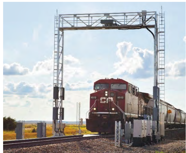
Figure 2. CPKC Train Inspection Portal System (TIPS), Maple Creek, SK
