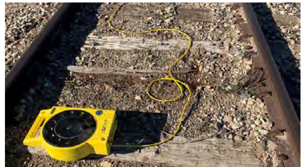
Figure 9. The track elevation is monitored using a ZipLevel which provides pressure feedback to the injection operator during polyurethane foam injection.
