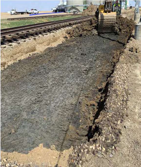
Figure 4. Subgrade susceptible to strength loss with freeze-thaw
