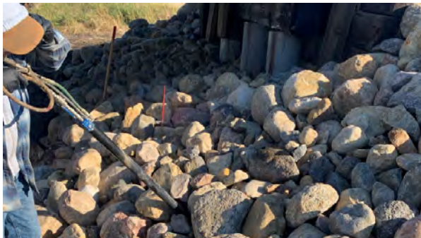
Figure 6. Following armouring and rip rap installation on East abutment wall, voids in the soil were injected with polyurethane foam.
