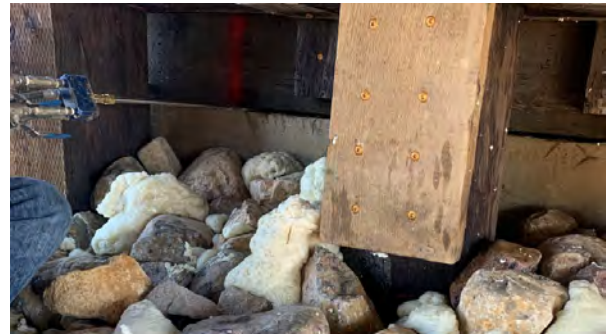
Figure 8. Polyurethane foam is injected into the backwall voids of the East abutment wall.
