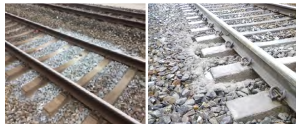
Figure 1. White spots of ballast breakdown (left) (Sysyn, et al. 2020) and Mud pumping induced by ballast fouling (right) (Nurmikolu et. Al (2013)
