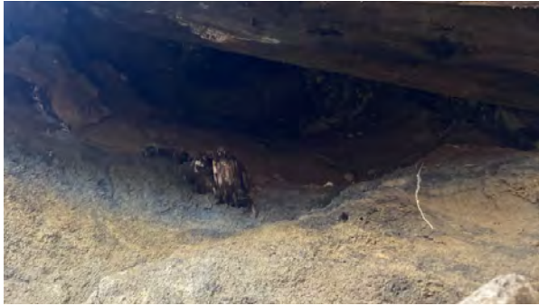
Figure 4. Following backwall and pile repairs, there were backwall soil voids that could not be filled or packed from above.
