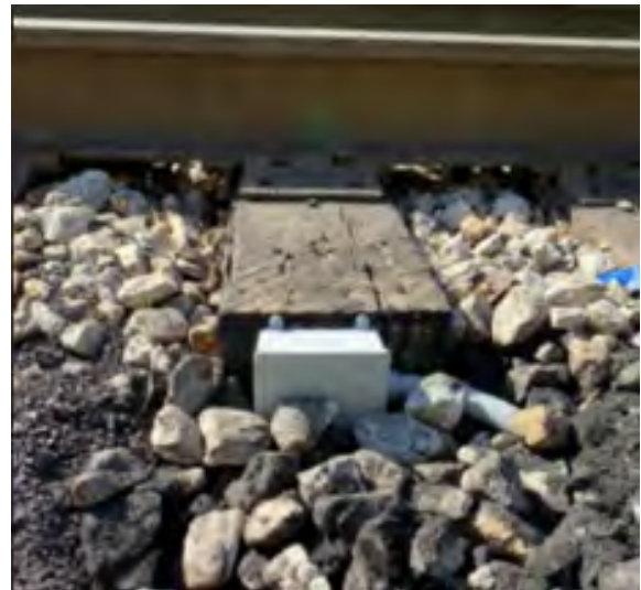
Figure 3. Accelerometer mounted on tie
