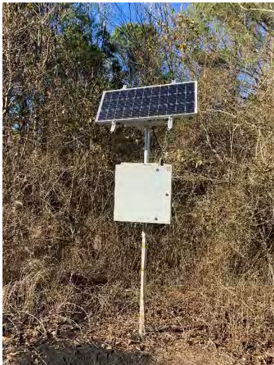
Figure 4- DAQ and Gateway enclosure
