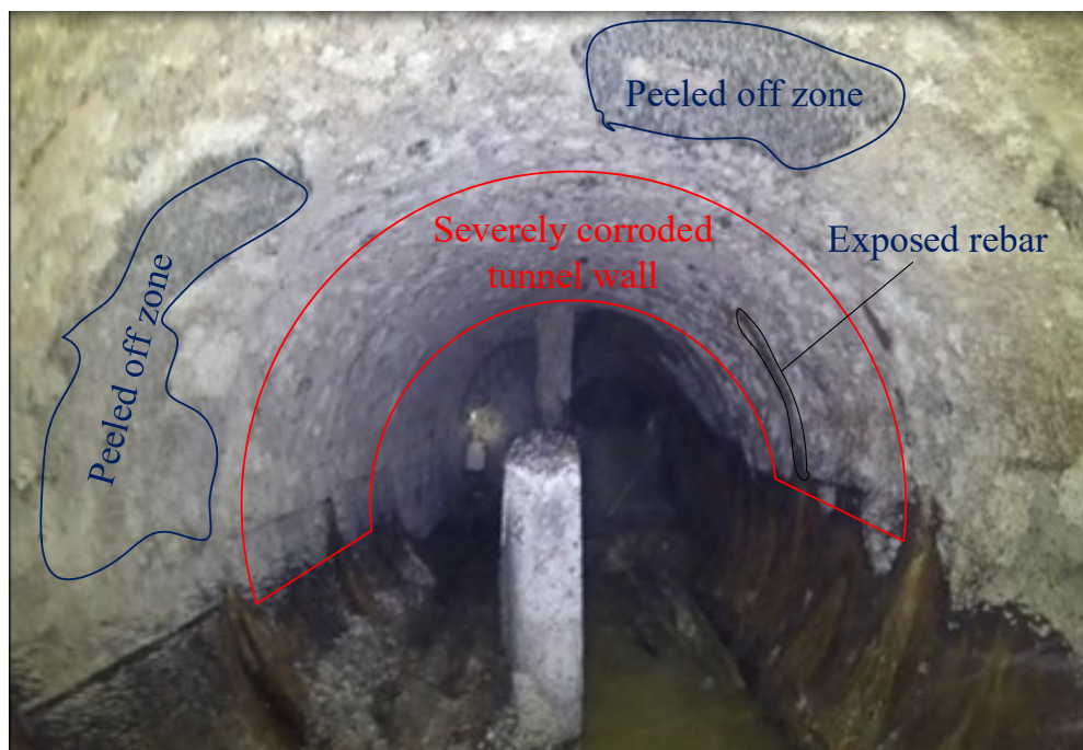
Figure 2.1. Corrosion conditions in a chamber located under the 127 street and 153 Avenue in Edmonton
