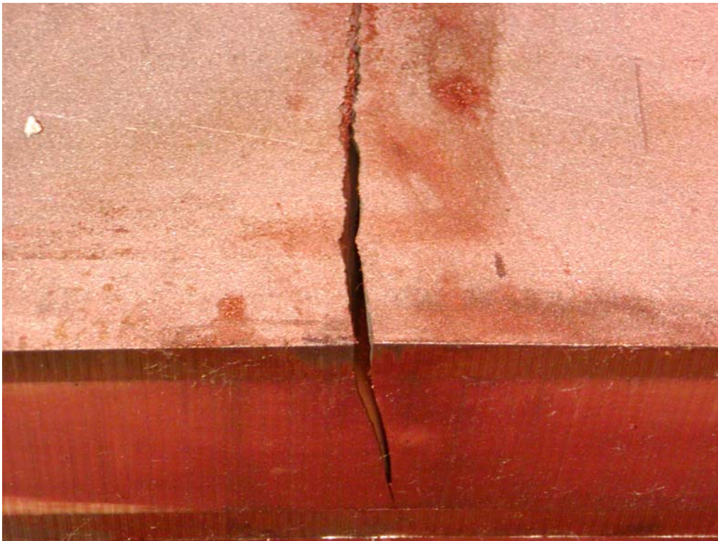
Figure 4.4: Fatigue failure of bottom steel plate (B5 shown).
