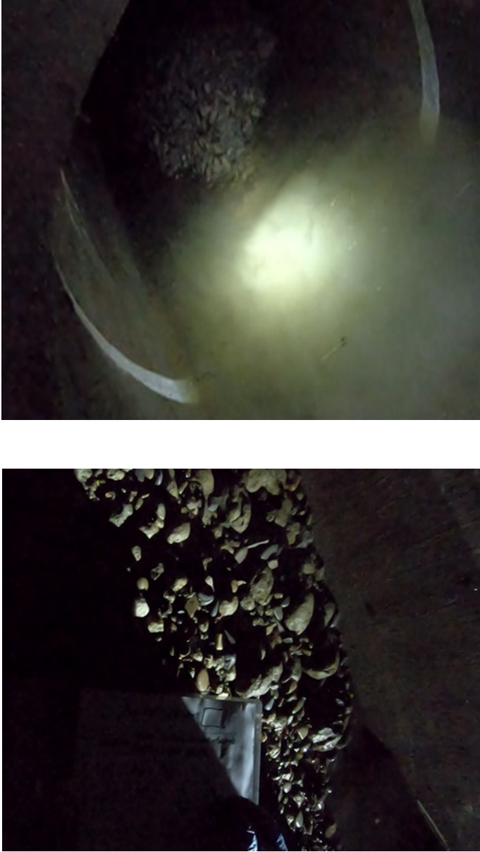
Figure 1-1. Significant amount of deposition in a storm trunk sewer
