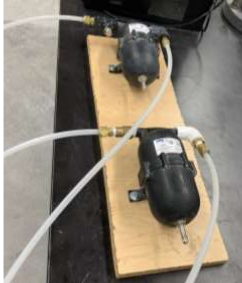
Figure 3-9. Dampeners added to the injection system.
