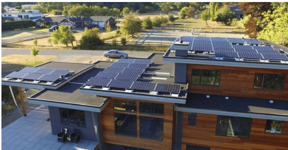
Figure 36, Solar Panel, (14kW Solar Panel Installation in Duncan BC n.d.)
