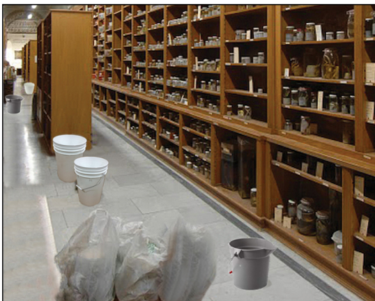
Figure 7. Multiple buckets placed to catch drips from roof leaks, as in the inadequately housed collection in Ottawa mentioned in the text.
