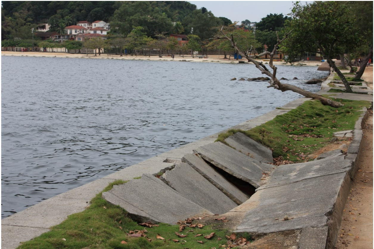
Figure 6. Holes in the sidewalk
