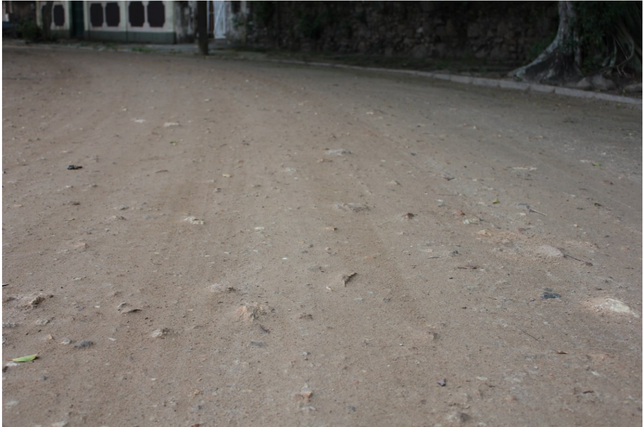
Figure 4. Gravel and holes due to rain
