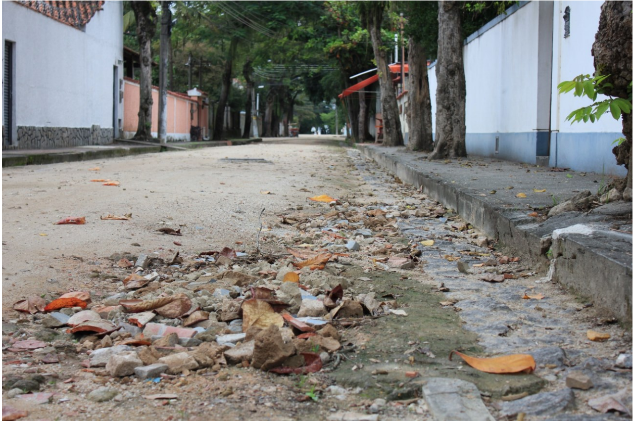
Figure 5. Rubble on the streets of Paquetá Island
