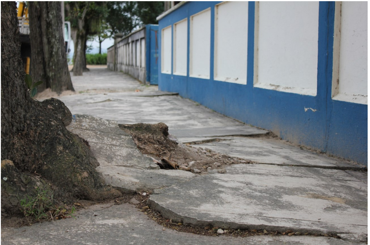
Figure 8. Sidewalks damaged by roots of a tree
