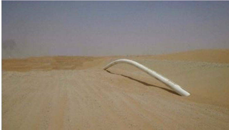
Figure 1-1: Upheaval buckling of a buried pipeline [6]
