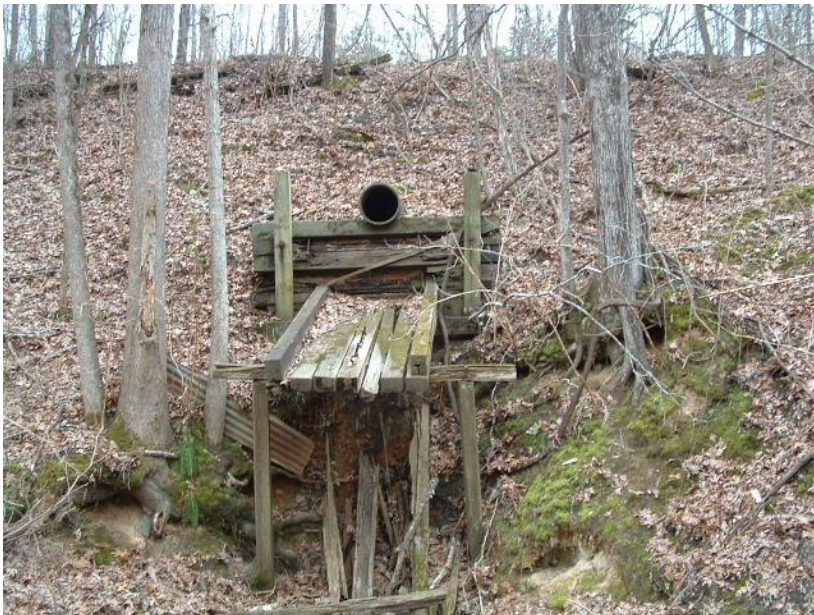
Figure A-8 This is the north side of the tunnel, the location was different than expected and thus we expect a kink in the result.
