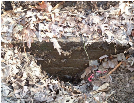
Figure A-17 This is the north side of the tunnel, it is partially filled
