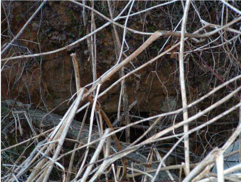
Figure A-14 The south side of tunnel 6, the tunnel was completely covered , but is not filled
