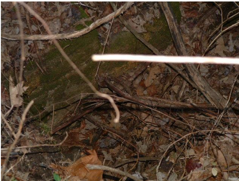
Figure A-15 The north side of tunnel 6, we cannot see if this part of the tunnel is filled or not.
