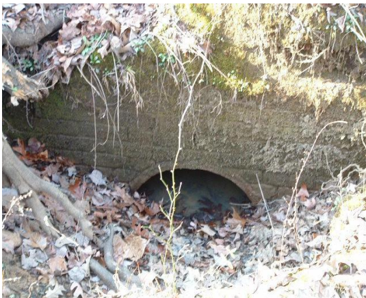
Figure A-18 This is the south side of the tunnel, there is a mixture of water, leaves and tree branches in the tunnel.
