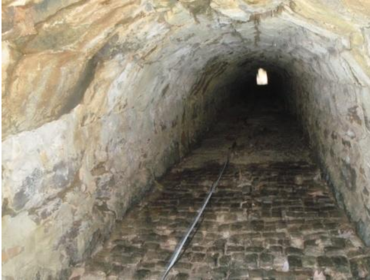
Figure A-1 This is the a picture of inside f tunnel 1. On the ground is a measuring tape used to put the 3-C geophones inside the tunnel during acquisition
