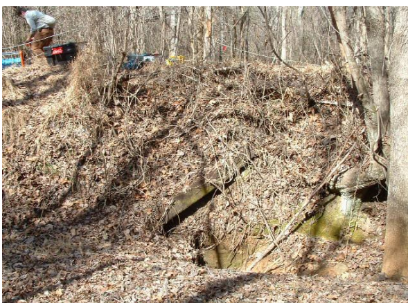
Figure A-13 , this is the south side of tunnel 5. The tunnel is partially filled.
