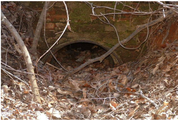
Figure A-12 , this is the north side of the tunnel 5, the culvert is partially filled
