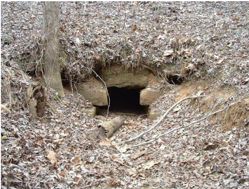
Figure A-10 This is the north side entrance into tunnel 4, this tunnel is created of concrete blocks and is approximately 0.5m.x0.75m.
