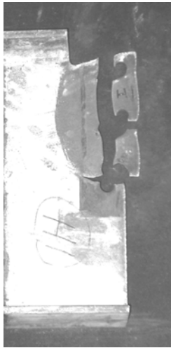
(n) Connection H1
