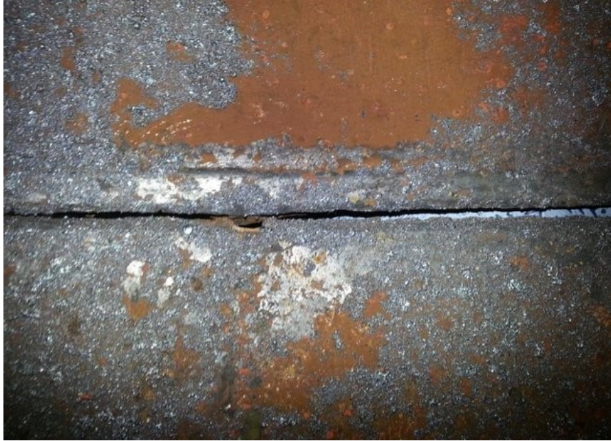
Figure 5: A photograph of a crack in a pipe [23].
