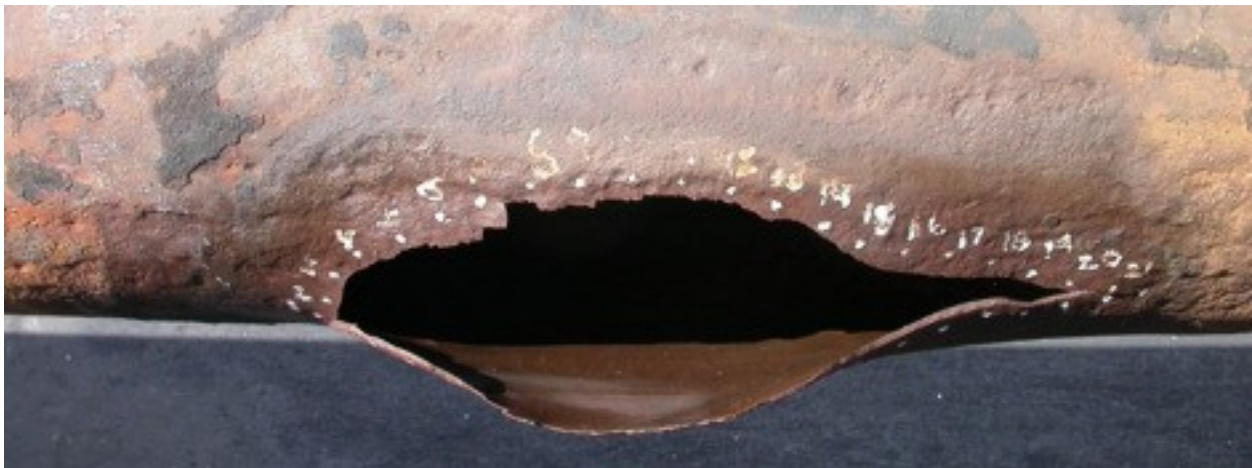
Figure 11: Uniform / General corrosion [35].
