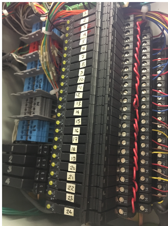
Figure 3.16: Solid state relays for test rig actuators. Pin layout is available in Appendix C.
