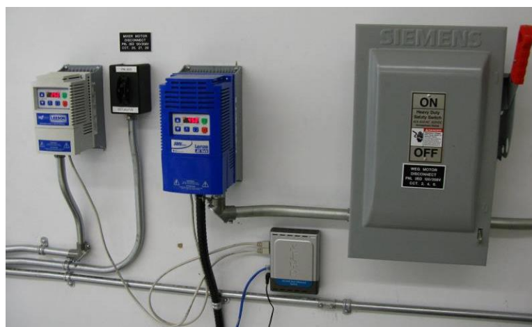
Figure 14 - VFDs for mixer (left) and pump (center); network switch at bottom
