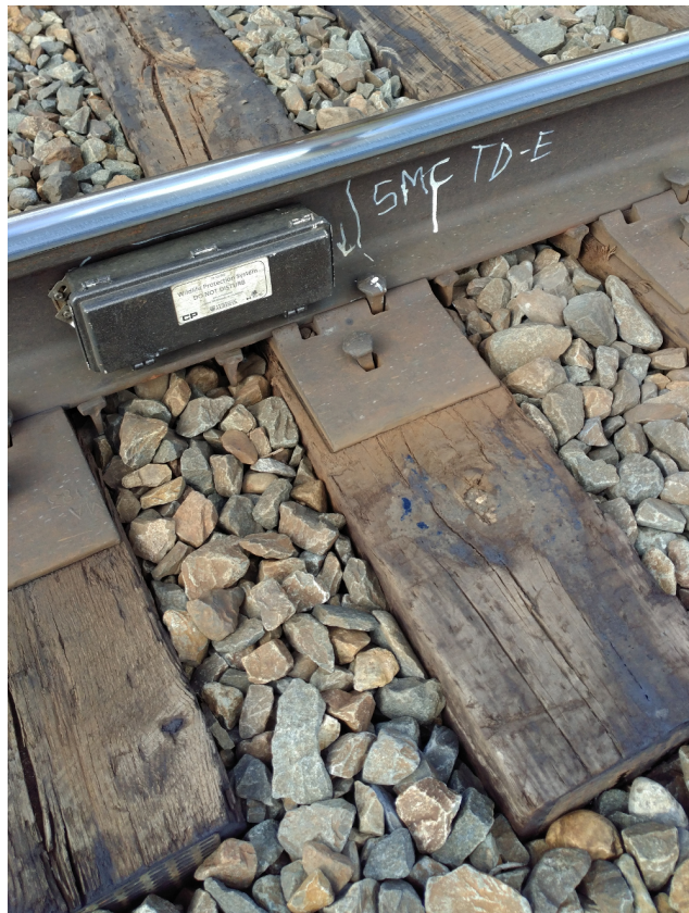
Figure D.3: Photograph of the box enclosure (a train detector) attached to the railway track.
