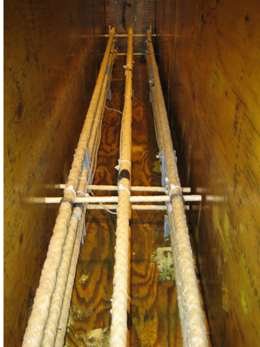
Figure C-4: Rebar cage positioned in the 600 mm deep formwork (specimen B6H). The No. 3 transverse support bars seen in the center of the photograph are located at mid-span. Similar support bars were provided at both ends.
