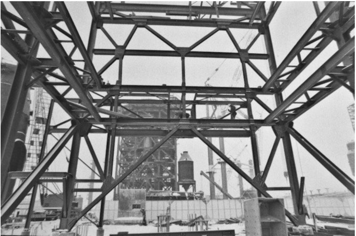
Figure 12: "Construction of the Syncrude plant," unknown photographer, Alberta (Winter 1976), 35mm negative, Imperial Oil Archives, IP 65, GA.
