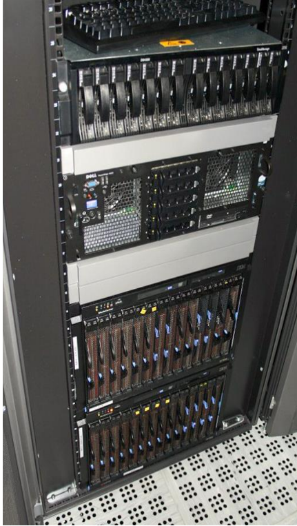
Figure 2 A standard 19-inch Rack
