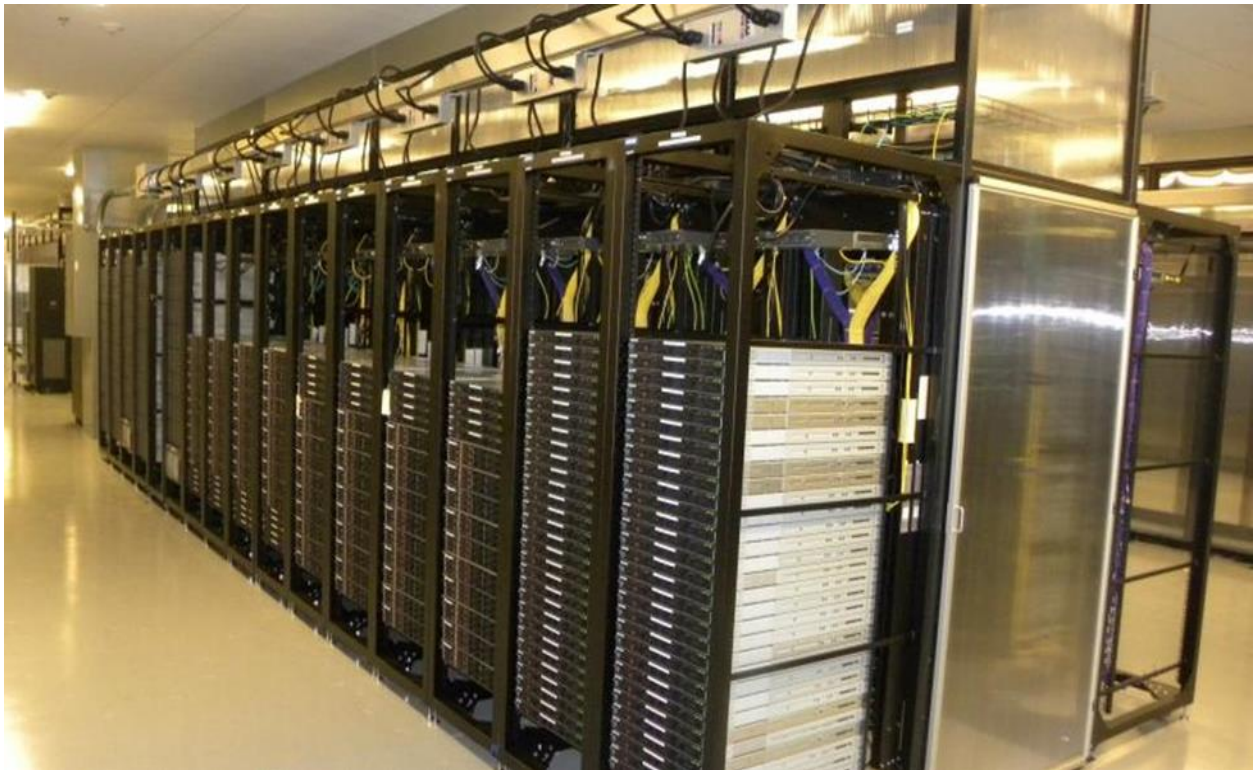
Figure 1: A layered, traditional data center setup on white space or physical facility.
