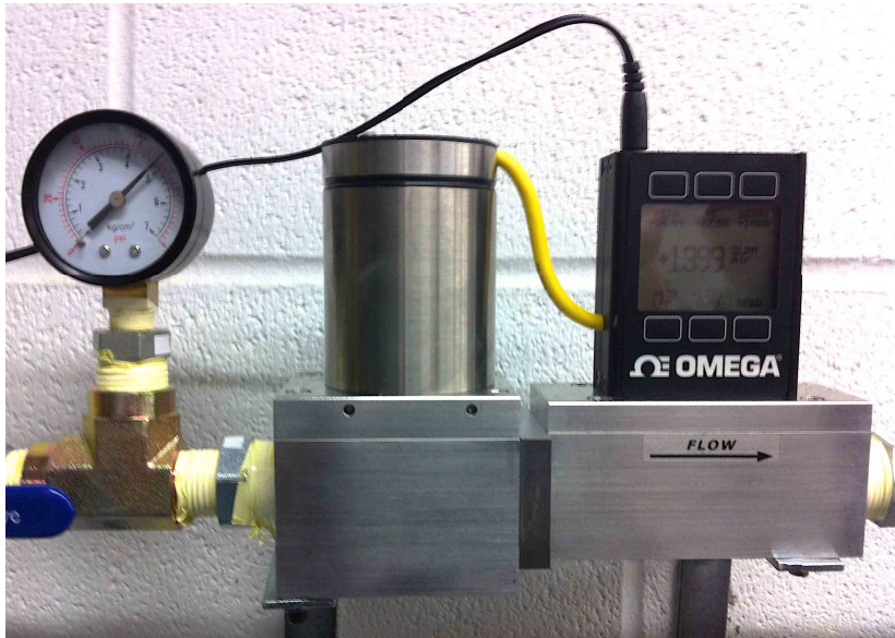
Figure 3.12 Mass Flow Controller for Air.
