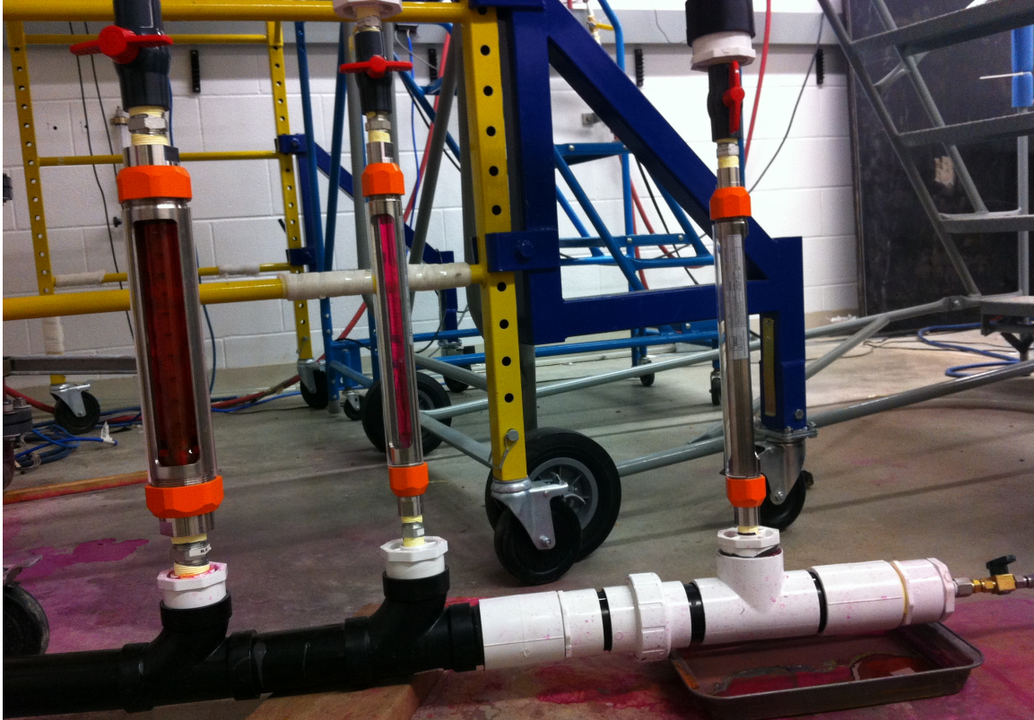
Figure 3.11 Three Water Rotameters with Isolation Valves.
