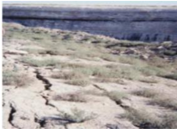
Figure 3: Cracking (Sankar, n.d.)
