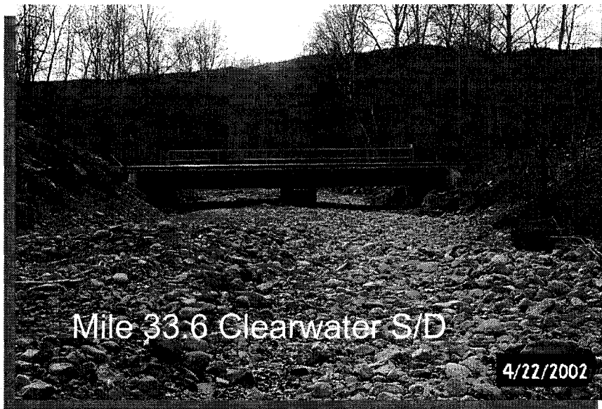
Figure 11-24 Case example of a Channel Aggradation / Debris Flow - Avulsion - Local Scour / Seepage Erosion / Gully Erosion hazard scenario initiating with an aggradation hazard event at Mile 33.6, CN Clearwater Subdivision (photos by Tim Keegan, CN file 4670-CLR-33.6)
