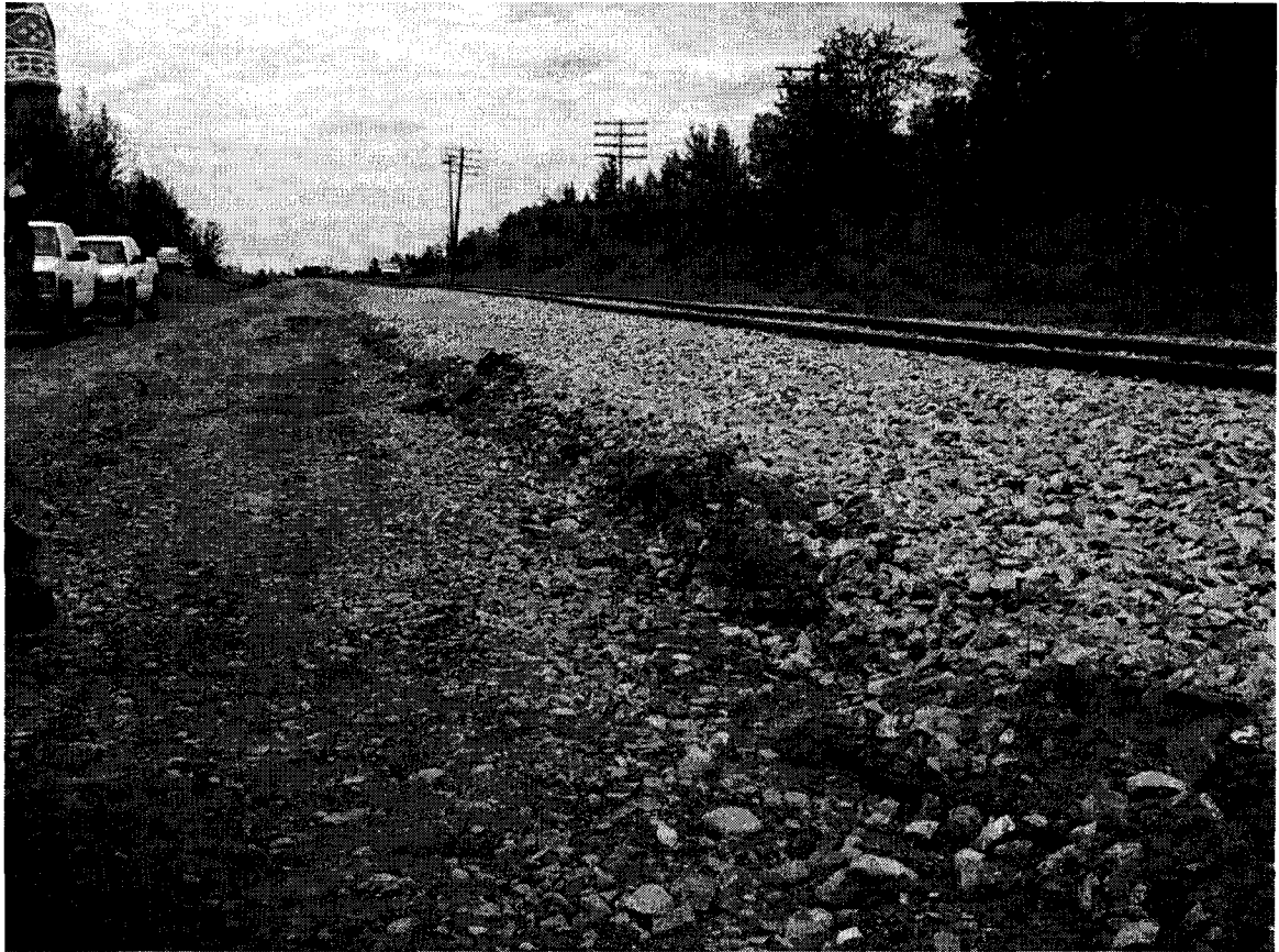
Figure 9-12 Illustration of a mud ridge and settlement caused by a subgrade plastic deformation event at Mile 67.6 CN's Edson Subdivision near Evansburg, Alberta (photo by Tim Keegan taken June 27, 2002, CN file ref 4670-EDS-67.6).
