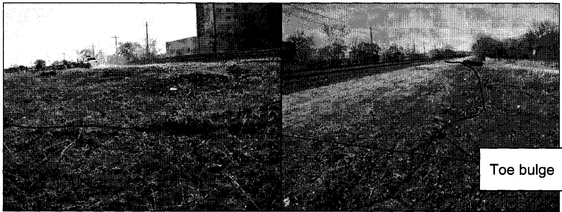
Figure 8-21 Case example of an earth slide caused by seepage from a ballast trough at Mile 0.6 of the CN Rivers Subdivision, Winnipeg, Manitoba (Photos by Tim Keegan on April 24, 2006, CN file 4670-RVR-0.6-1.0)
