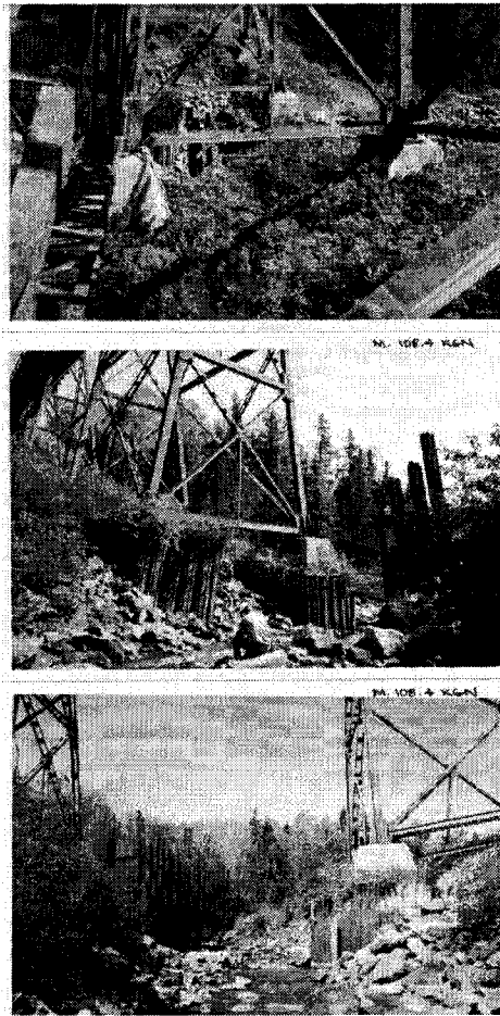
Figure 11-28 Case example of a General Scour / Channel Degradation – Earth Slide hazard scenarios Mile 108.4, CN Kinghorn Subdivision (photos by Tim Keegan, CN file 4670-KGH-108.)
