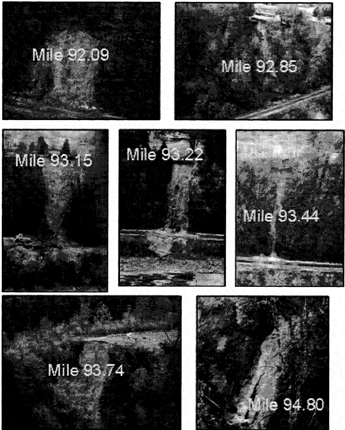
Figure 8-6 Typical Earth Slide- Earth Flow hazard scenarios @ Mile 92 to 95 of CN's Yale Subdivision where simultaneous Earth Slide-Earth Flows from the upper slope caused track failure (track blocked). (Photos taken by Tim Keegan Sunday, September 05, 2004, CN file: 4670-YLE- 92-95, (BGC, 2004)).
