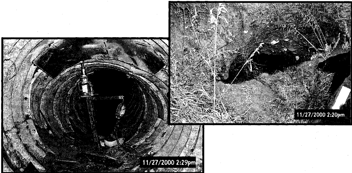
Figure 10-10 Photos of pulled apart culvert (left) and collapse feature (right) as an example of a preparatory cause for a Seepage Erosion / Piping - Earth Slide hazard scenario. (Mile 148.22 CN Wainwright Subdivision, photo by Tim Keegan, CN File 4670-WWR-148.22)
