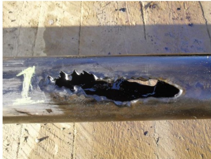
Fig. 2-5. Example of eroded tubing from MacKay River SAGD project [14].
