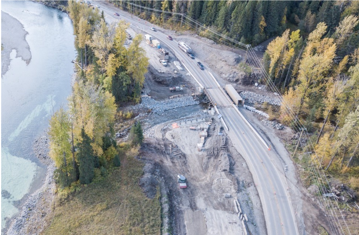
Figure 7-6. A $6.3M Highway 3 bridge replacement over Lizard Creek, near Fernie, BC, taken summer 2019. This bridge replacement includes an engineered wildlife underpass.
