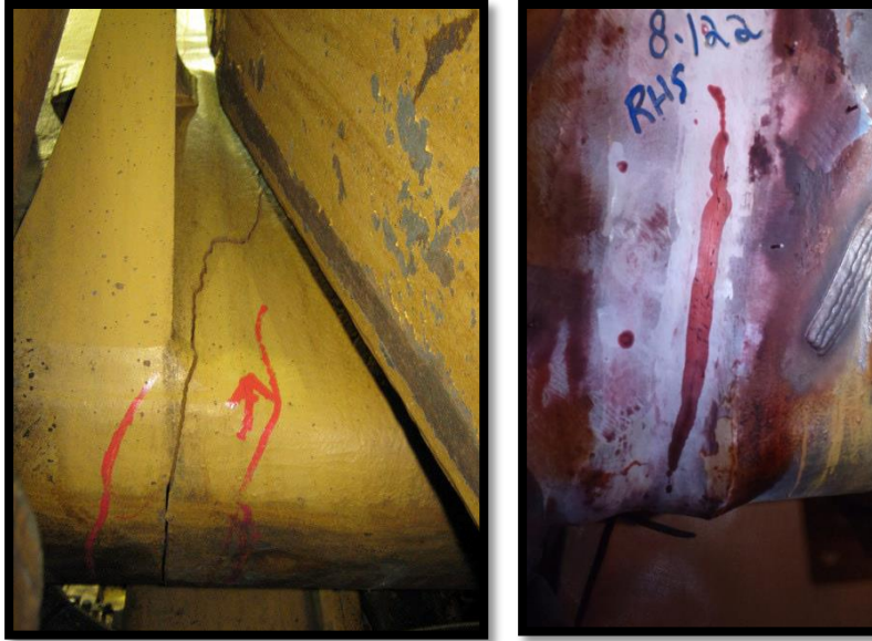
Figure 2.24 Frame crack (Truck A on the left and C on the right) (Amarra & El-Sayed, 2010)
