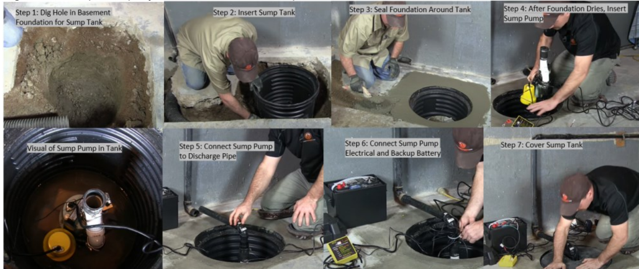
Figure 2: Sump Pump System Installation Example
