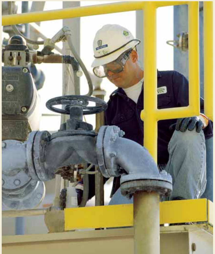
Fred Cutler, PAP Operator, checks equipment at our Aurora purified phosphoric acid facility.
