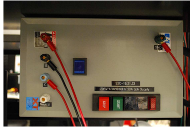
(a) Connector box to the three-phase power source
