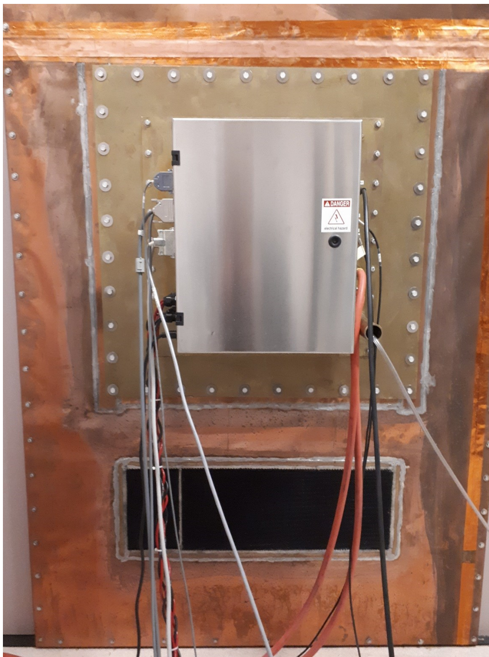
Figure 2.14: Filter panel at the back of the vault for shim, gradient, RF, and lighting cables, as well as water cooling lines.
