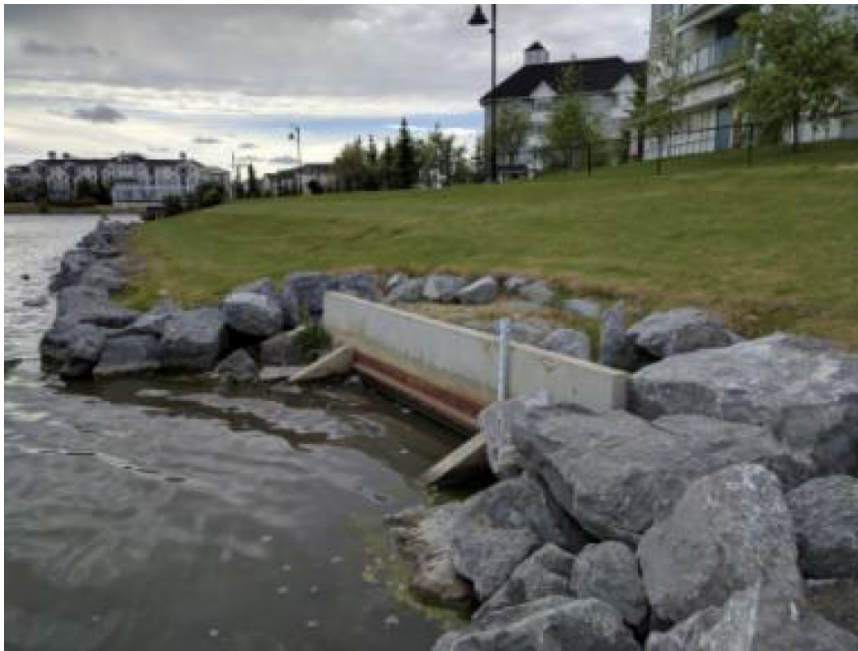
Figure 0-5: Sampling site WP31C located in Country Hills Stormwater Facility.
