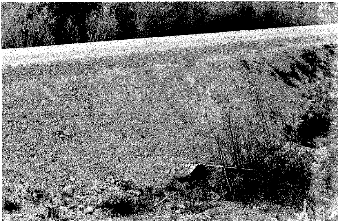
PLATE 1 : Reconstructed embankment, about 5m. high. Original culvert is slightly below ditch level and contains remnant aufeis (Kilometer 6).
