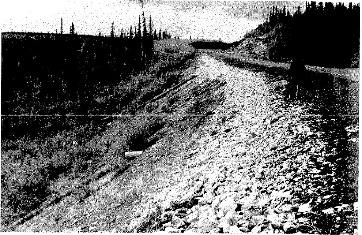
PLATE 9: Sideslope 16 m. high fill at 34 degrees to the horizontal. (Built 1976). Culvert in foreground collapsed. "Fluming" is intact (foreground).
