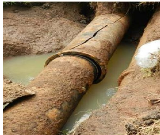
(c) Inclined crack
