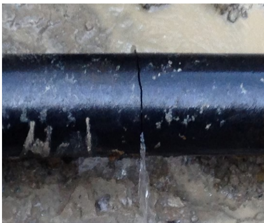
(b) Circumferential crack
