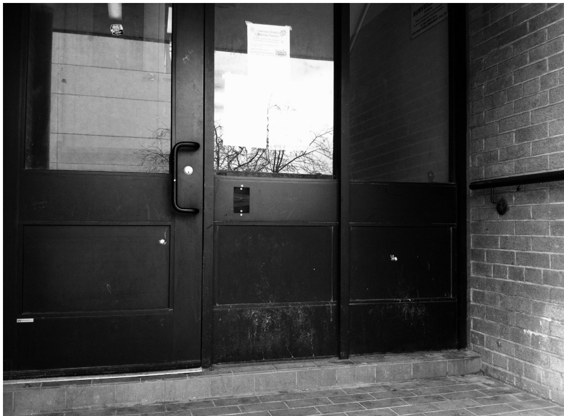
Figure 8: Back of Building on Amaranth, Post-Shooting: Note the patched bullet holes on the door handle, below the handle, and to the far right. TCHC was forced to replace the glass.
