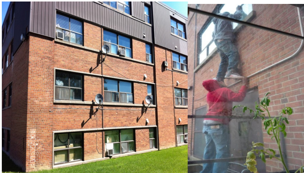
Figure 6: The Outside of a 4-Storey Building and Break-and-Enter in Progress
