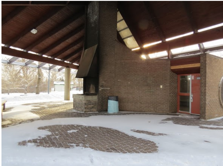
Figure 20: An image of the outdoor fireplace located in a public park next to the river. Image taken February 9, 2017
