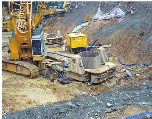
c) Lift Casing
