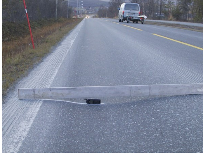
Figure 1.3 An example of extreme rutting in a pavement structure [11].
