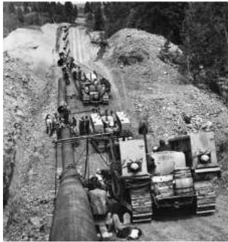
Figure 4: The above photographs display Terasen Pipelines building the Trans Mountain pipeline in 1953. This photo illustrates the challenges of building pipelines.
