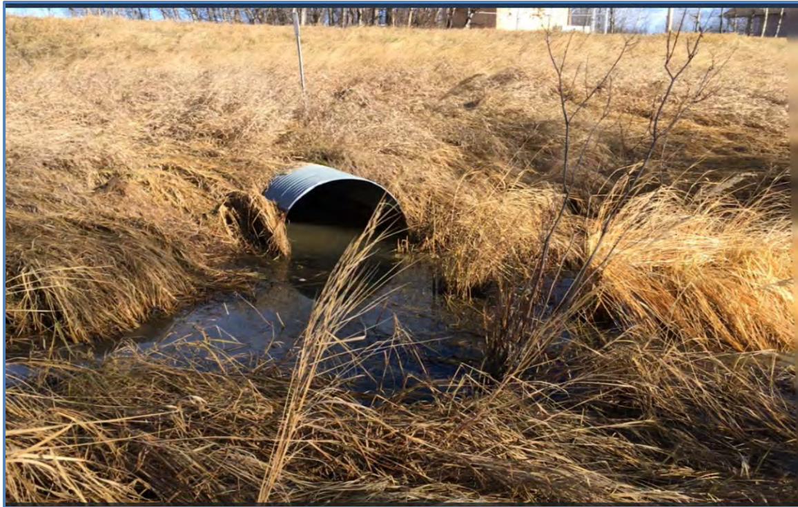
Figure 4.5b - October 24, 2017, Photo Showing Vegetation and Standing Water Restricting Outflow at Downstream End of Antler Lake Outlet Culvert.
