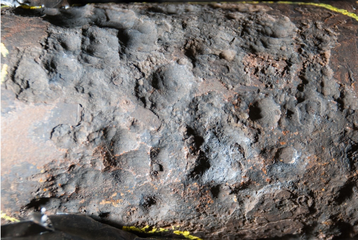
Figure 5.1 Presence of tubercles in conjunction with pitting degradation driven by MIC in a carbon steel tubing subjected to intermittent produced water flow.
