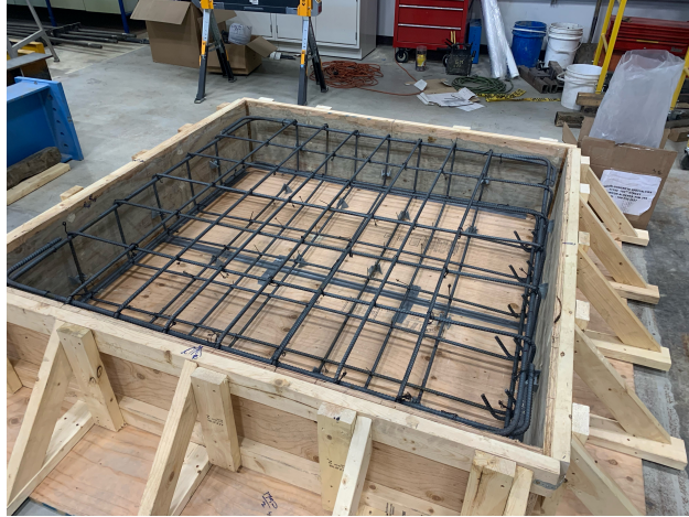
Figure 5.3 – Reinforcement cage prior to embed placement and concrete pour (lifting hooks not shown).
