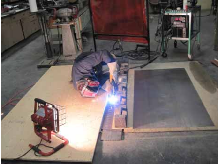
Figure 6-10: Welding Infill Panel Lap Splice Joining Two 20 Gauge A1008 CS Steel Sheets
