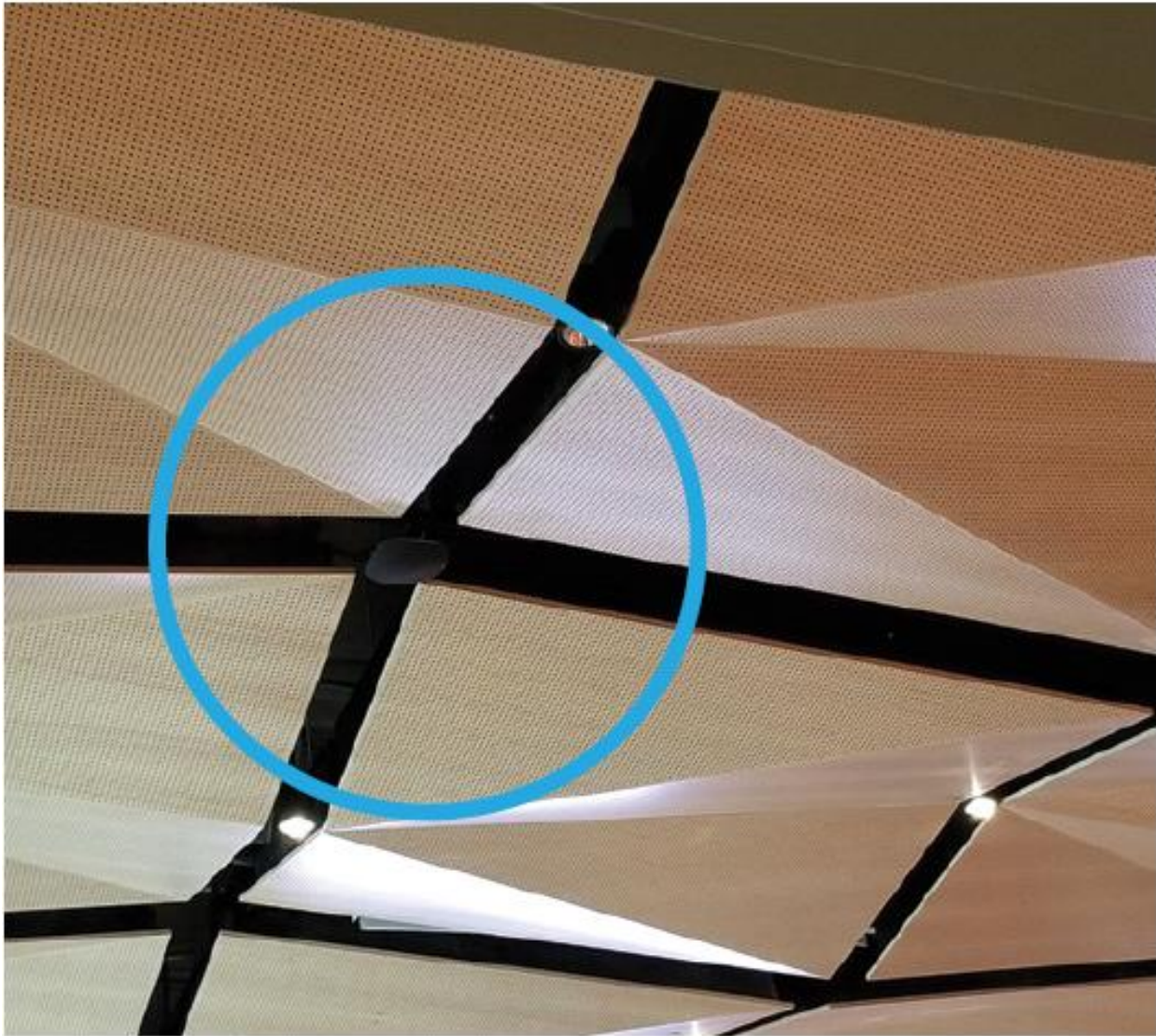
Figure 28 Example of an AP deployment within an intelligent building ceiling designed for aesthetics. The goal accomplished is to hide the AP. [20]
