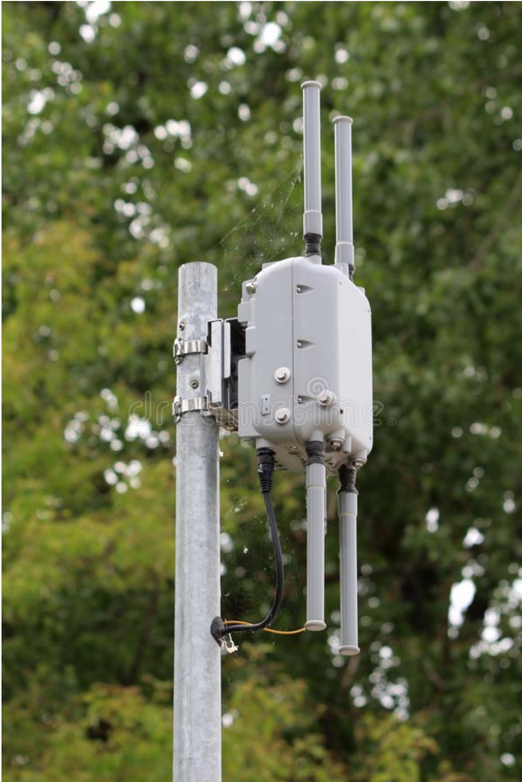
Figure 29 Outdoor Access Point mounted on a pole [48]
