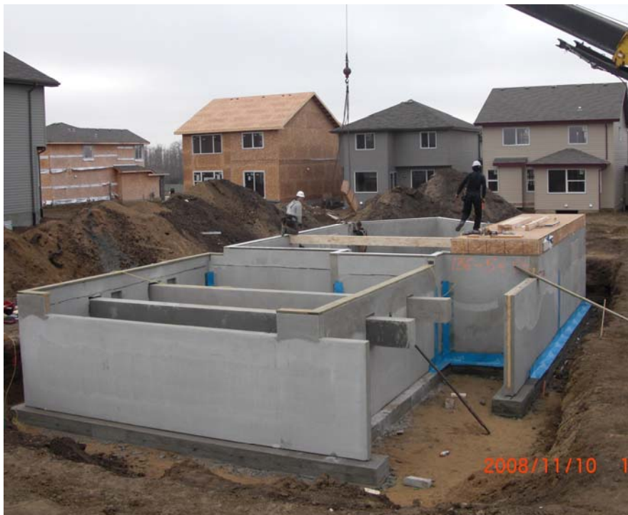
Figure 5-14: Sandwich Panel Foundation (07-133)
