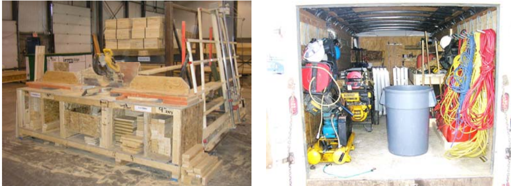
a. Cutting Station for Floor Prefab Cell b. Tool Trailer of a Field Erection Crew
