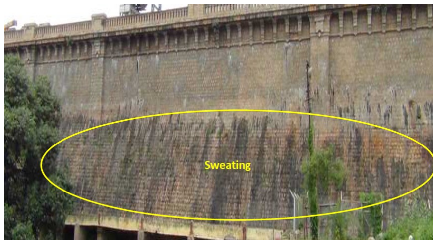
Figure 1.2 Seepage through Body of the Dam in the form of Sweating
