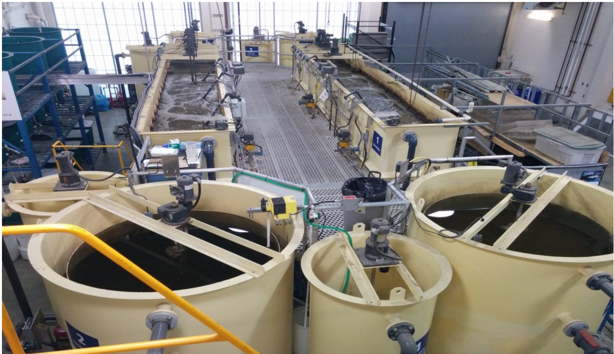
Figure 2 Image of Twin pilot-scale plant at EPCOR's Goldbar Wastewater Treatment Plant
