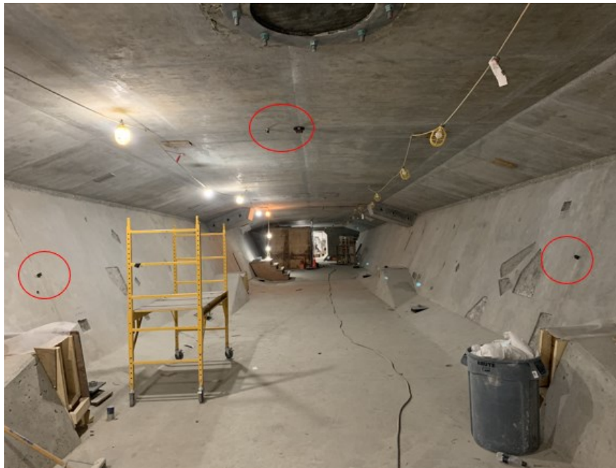
Figure 3.4. G-Link-200 (circled for emphasis) installed inside box girder
