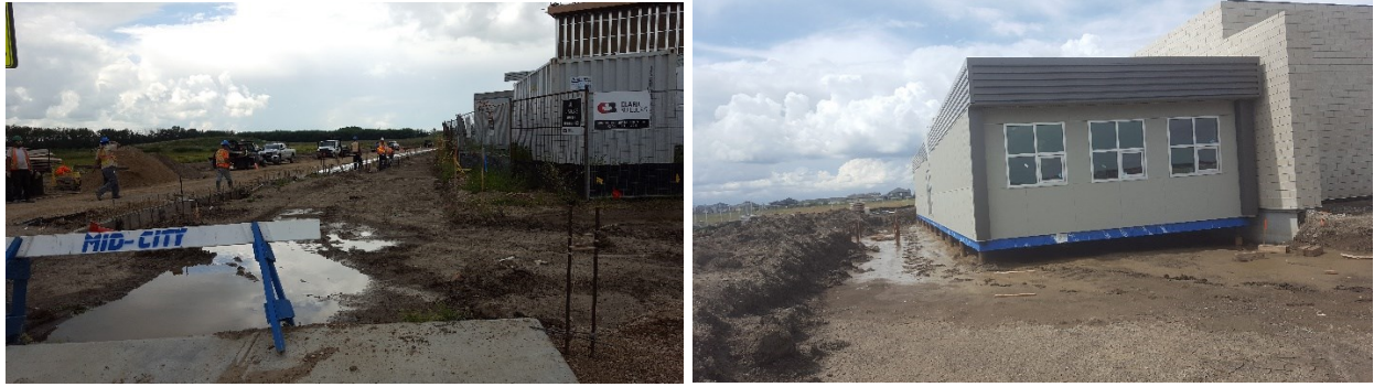
Figure A- 15.Flooding at the time of installation
