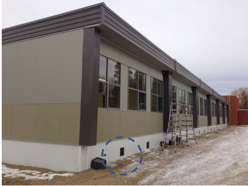
Figure A- 5. Ventilation ducts below the units
