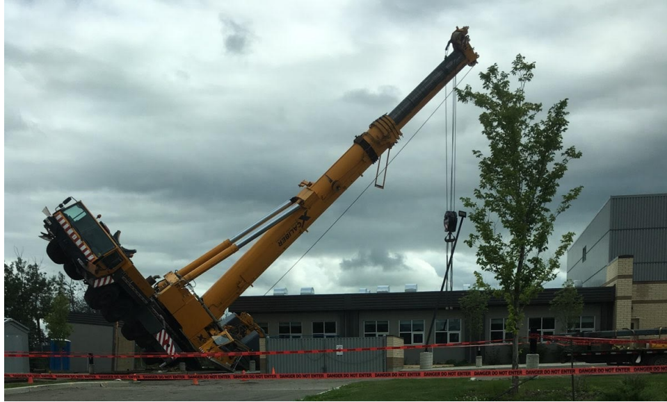
Figure A- 17. An incident during the installation of a module
