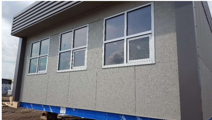
Figure A- 13. A broken window at the transportation stage
