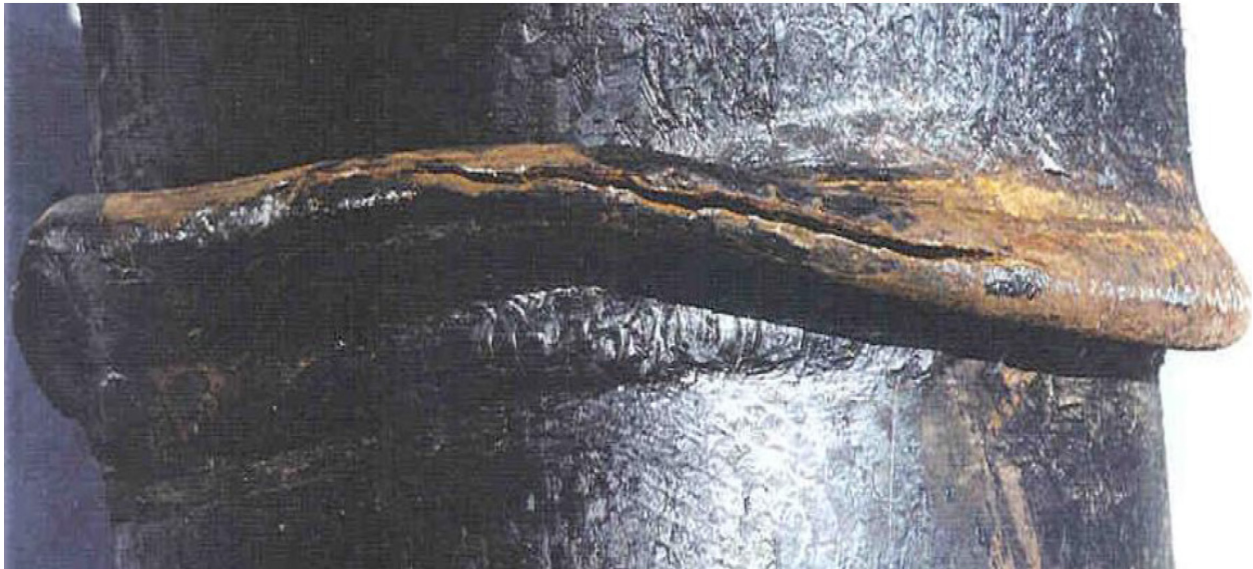
Figure 2- 1:Wrinkle formation near a girth weld and the resulting cracking of pipe wall at the apex of the wrinkle (Wang et al. 2017).
