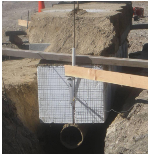
Figure 2- 11: Photograph of the end of the trench, pipe, EPS block after the uplift test (Bartlett and Lingwall 2014).
