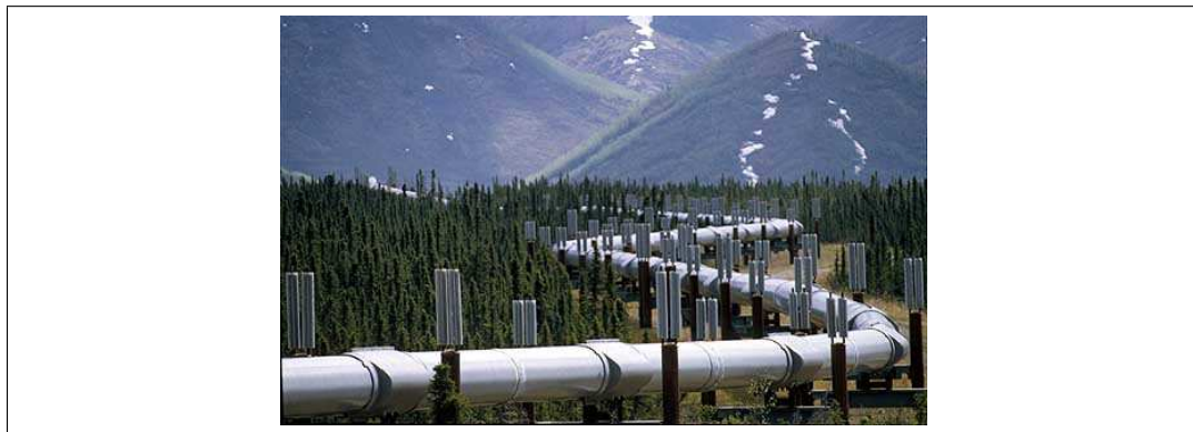
Figure 1.5: Using ultrasonic sensors for corrosion monitoring of the Trans-Alaska oil pipeline.
