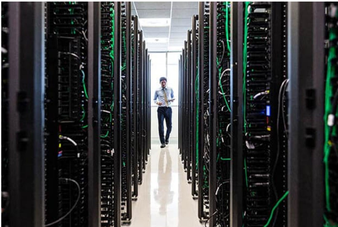
Figure 1 Traditional Data Center ii
