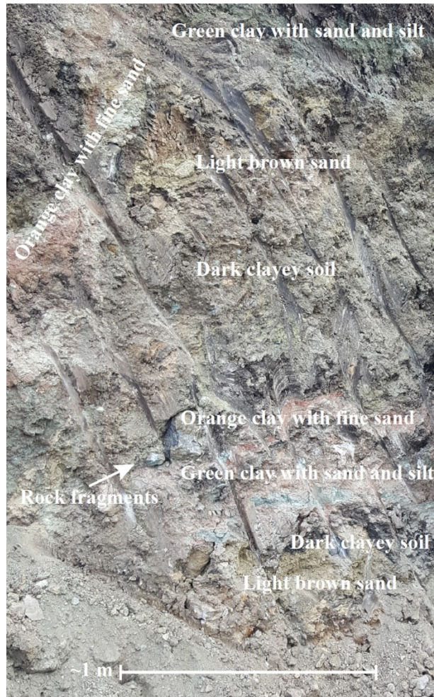
Figure 5-2 Photographs of the earthflow showing the churned strata from a cut adjacent to the access road located between the highway and the railway at the Ten-mile landslide (October 2016).
